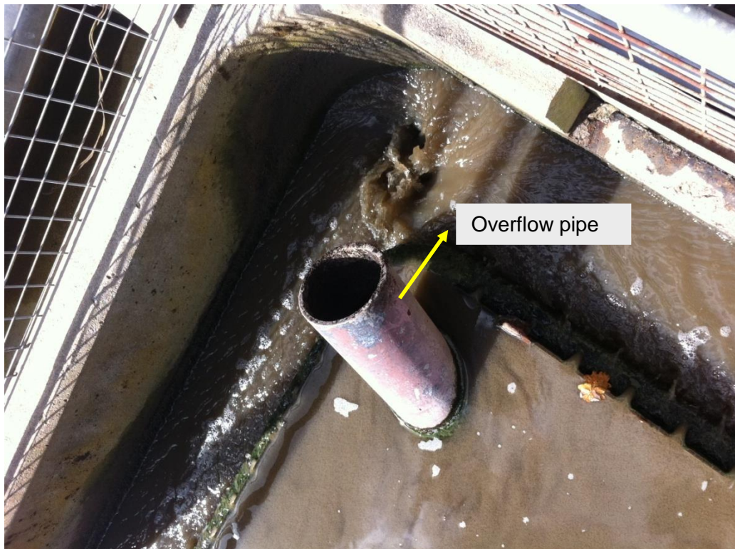
Figure 4.2 Photo STP Aerator Tank
