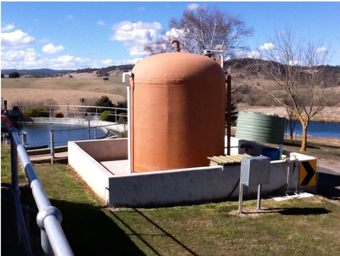
Figure 4.2 STP - Alum Storage Tank Bund
