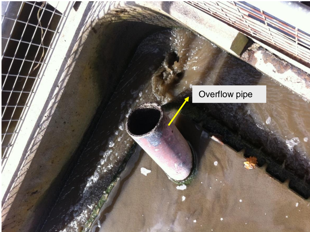
Figure 4.2 Photo STP Aerator Tank
