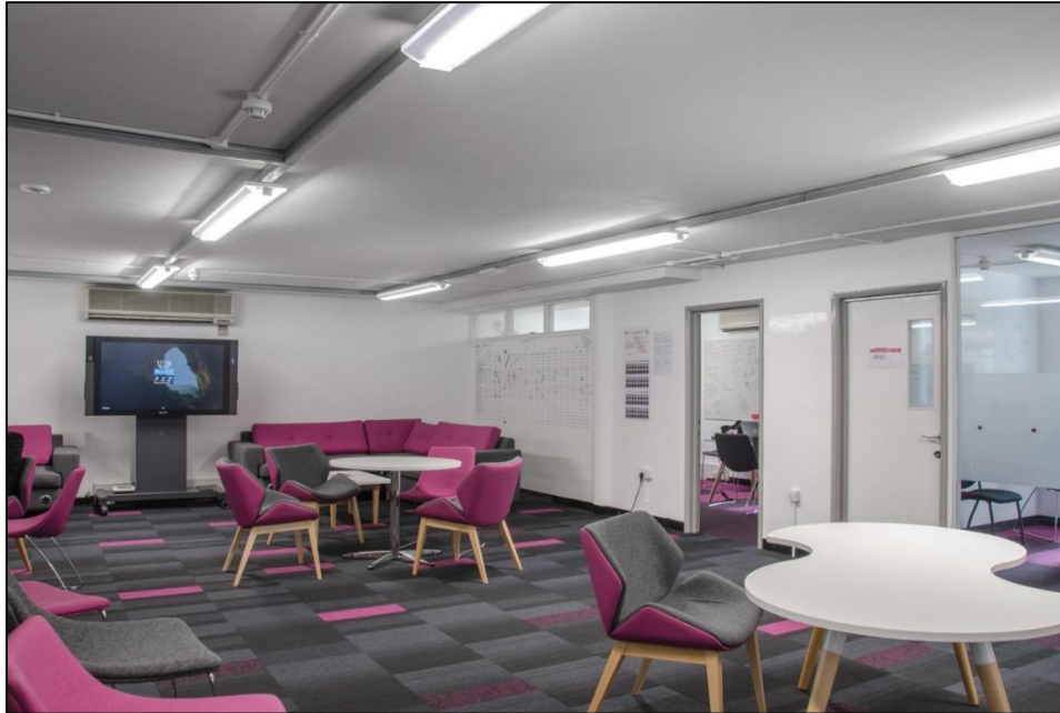
Figure 13: Example Thorlux LED Luminaire
