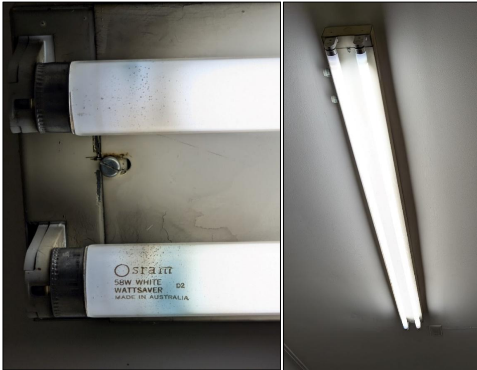
Figure 11: Council Admin Fluorescent Lighting
