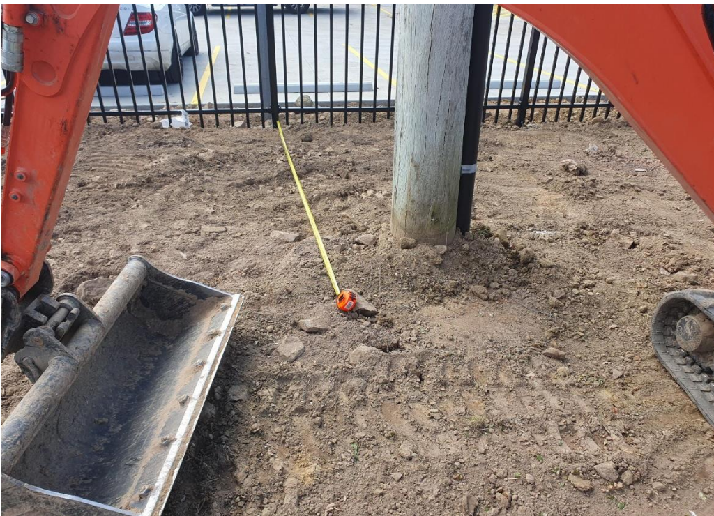
Figure 5: Tape measure showing 3.5 metres (Condition 31 requirement) from boundary fence to tape measure. Distance from fence to power pole is 3.05 metres. Therefore, clearance to edge of required pathway is 45 centimetres.
