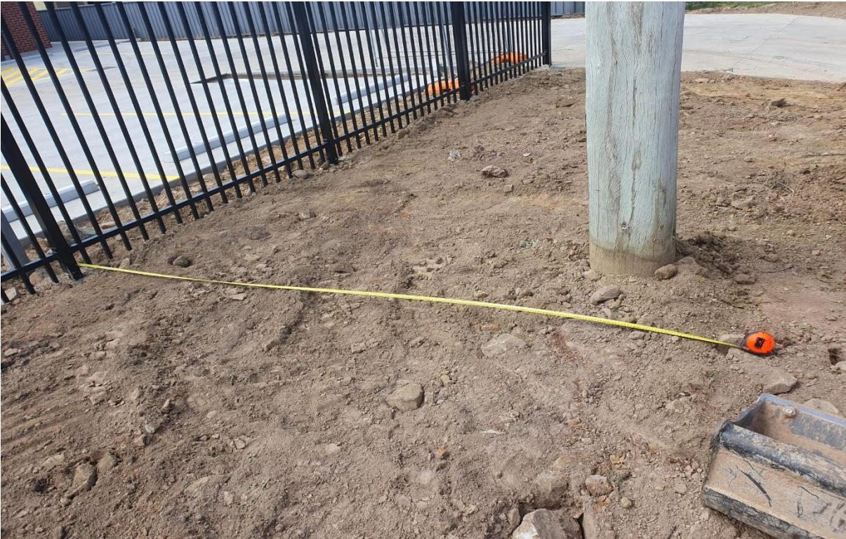
Figure 6 A pathway installed parallel to the front boundary would connect with the driveway.
