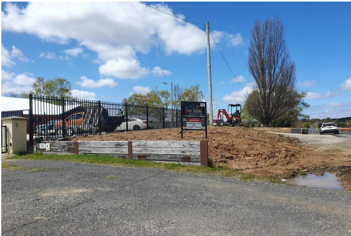
Figure 3 East view showing street alignment and retaining wall (max height 600mm) inset by 1.2 m from the carriageway alignment.
