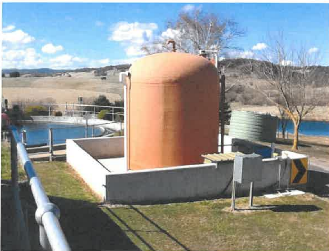
Figure 4.2 STP - Alum Storage Tank Bund
