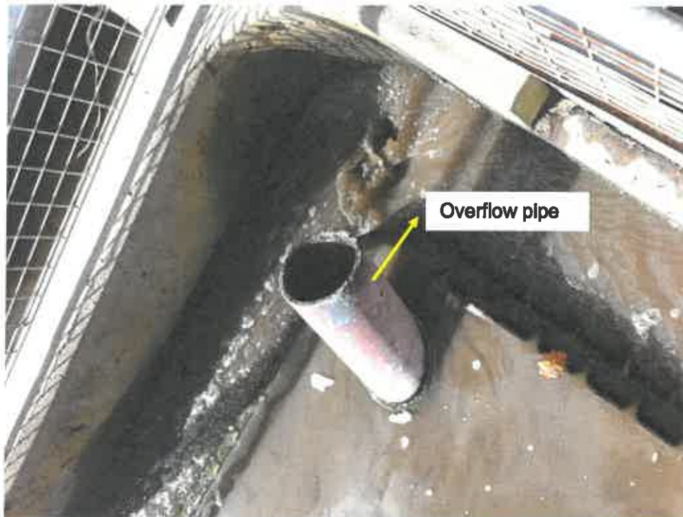
Figure 4.2 Photo STP Aerator Tank
