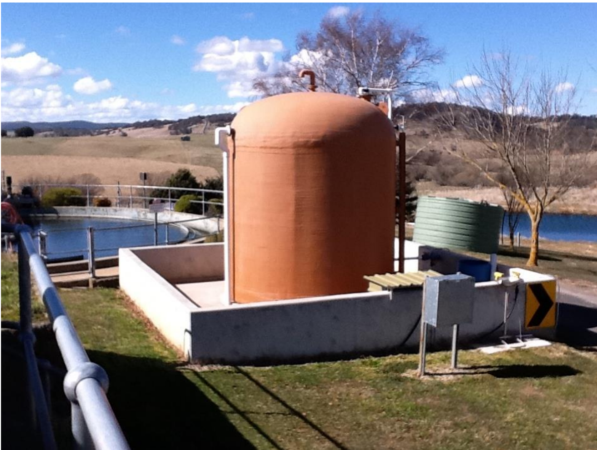
Figure 4.2 STP - Alum Storage Tank Bund
