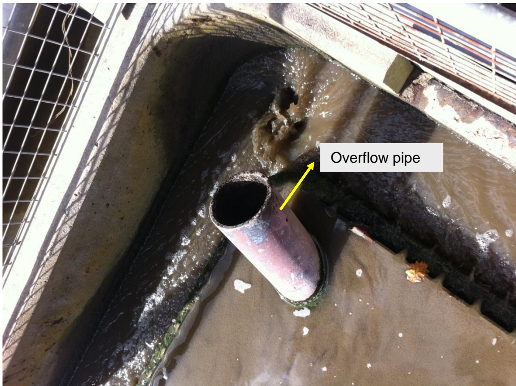
Figure 4.2 Photo STP Aerator Tank
