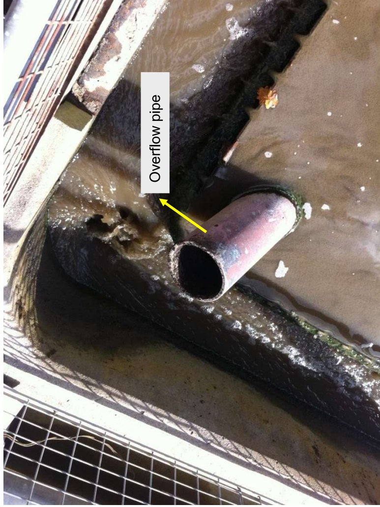
Figure 4.2 Photo STP Aerator Tank
