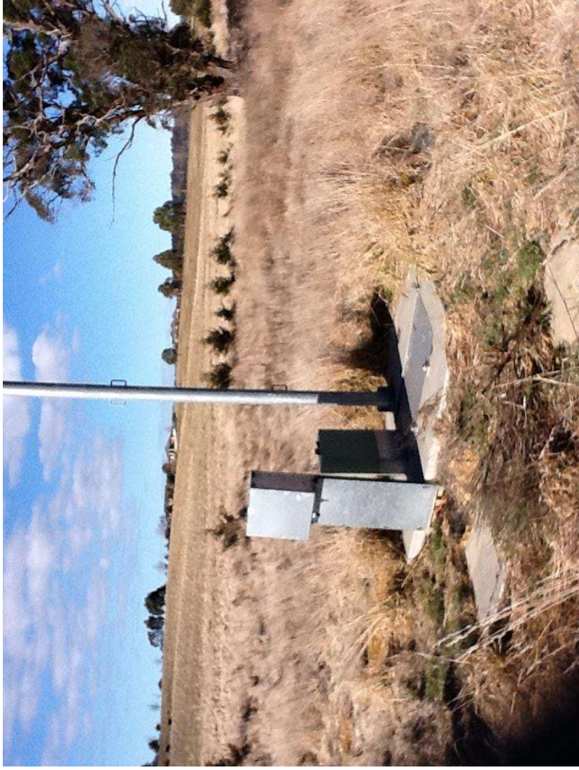
Figure 4.6 Photo SPS No.4
