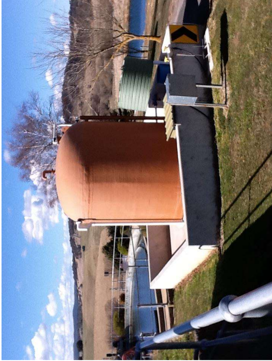
Figure 4.2 STP - Alum Storage Tank Bund
