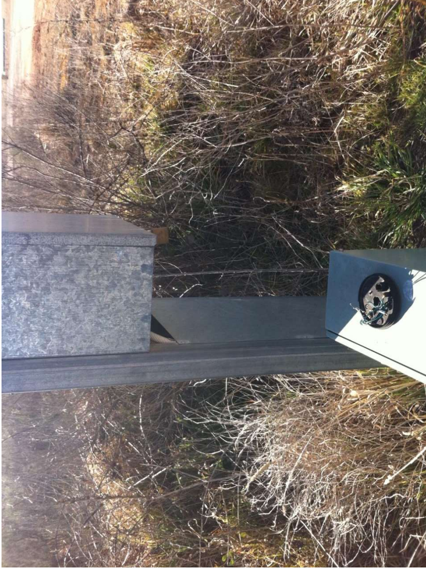
Figure 4.5 Photo SPS No.3
