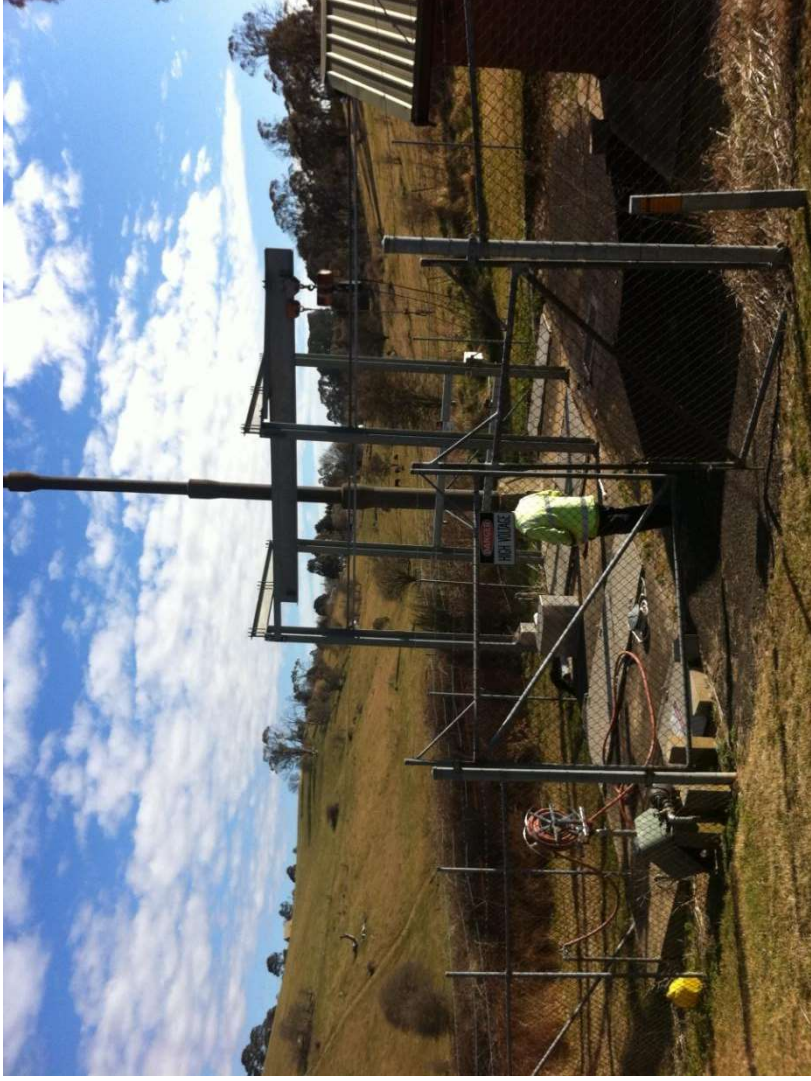
Figure 4.3 Photo SPS No.1
