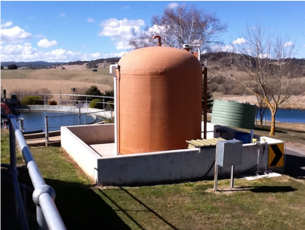
Figure 4.2 STP - Alum Storage Tank Bund
